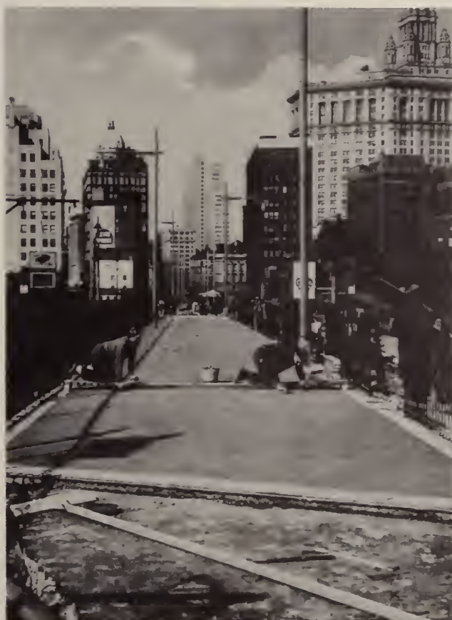
The promenade, as it passes over Franklin Street, receives a new concrete surface.
